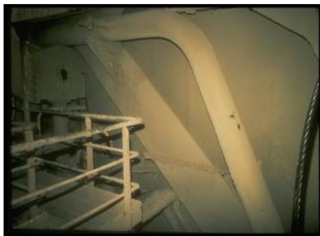
Figure 2 - Port diverter vent line (the identical starboard line failed in less than 10 minutes; the elbow wall thickness was 3/4 in.)
